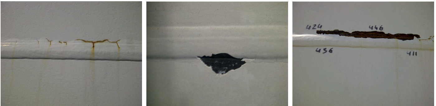
Examples of affected welding seams caused by rust
